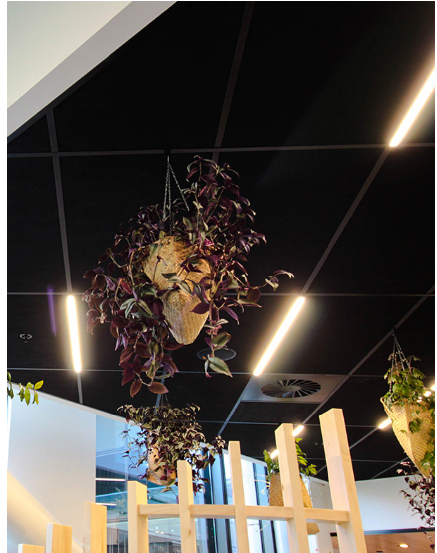
Figure 22. C Max Absorb and GridLux Lights installed in Koha Gym.
